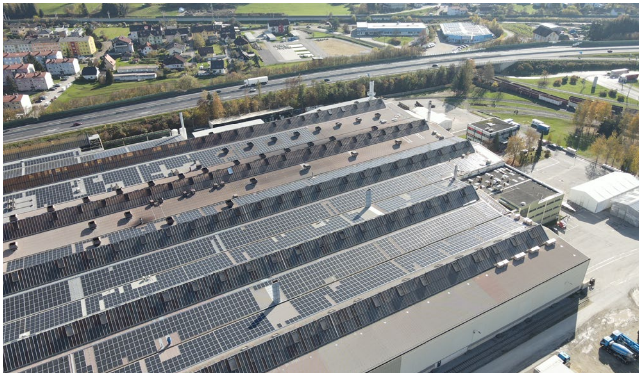
Fig.: PV system on the roof of the seamless tube rolling mill
