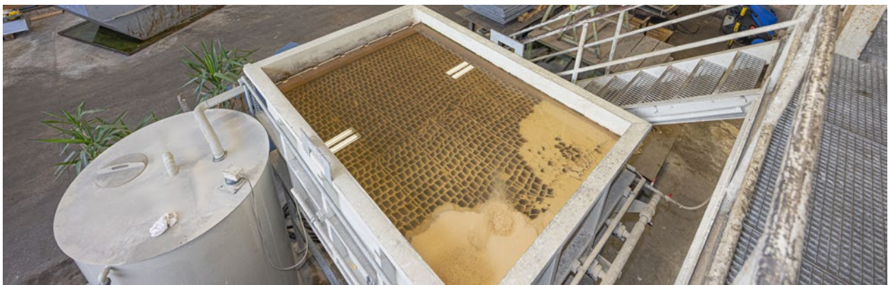
Fig.: Neutralization plant
