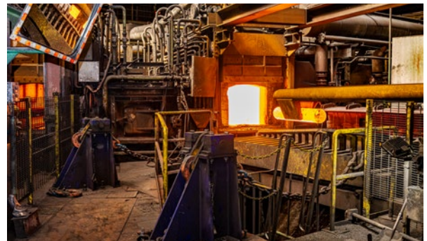
Fig.: Rotary hearth furnace
