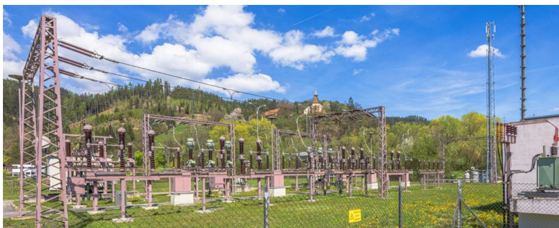
Fig.: Transformer substation
