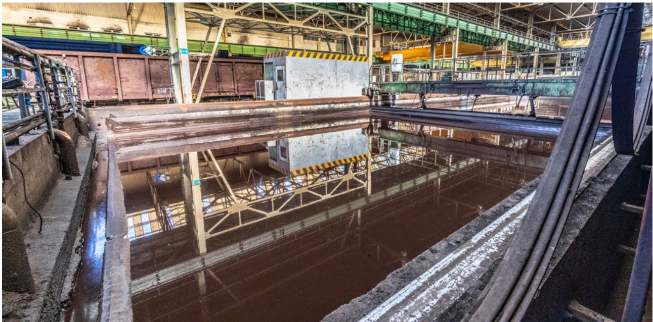
Fig.: Wastewater purification system for seamless tube rolling mill
