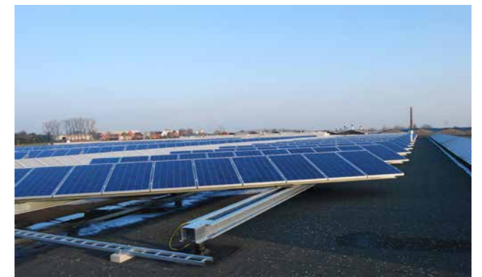
ROOF TOP SOLAR STRUCTURES
