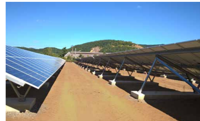
GROUND MOUNT SOLAR STRUCTURES
