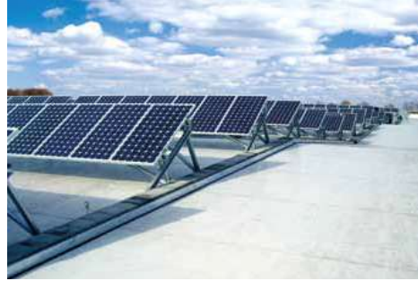
AS LINEAR SPREAD LOAD (resting on the support structure of the building)
