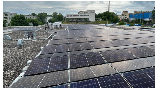
124,67 kWp, gravel roof eco-tec.at Photovoltaics GmbH
