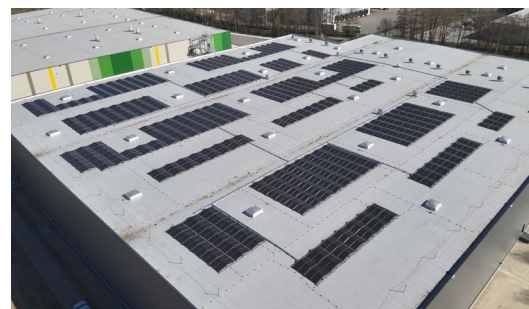
557 kWp, tetto in laminato SUNKON GmbH
